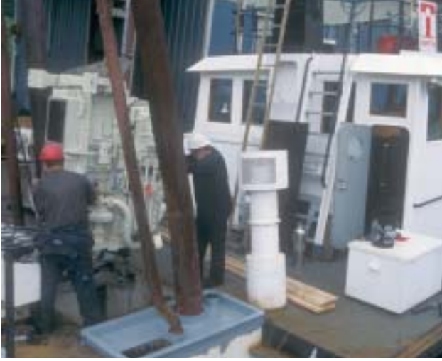
Island Tug and Barge's maintenance crew lowers one the new Cummins diesels through a hatch in the top of the Island Crown's fiddle. The engines, lifted with a specially-designed jig, were stood on their head to fit through the hatch with mere inches to spare.
